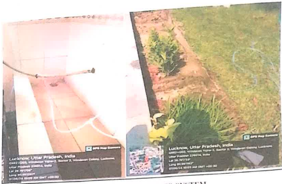
REUSE OF RO WASTE WATER SYSTEM
